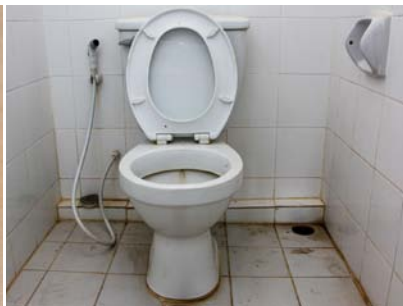
Water in toilet seat
